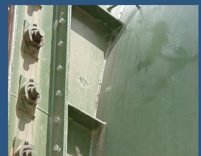
This picture shows the cracks found in the fan housing
